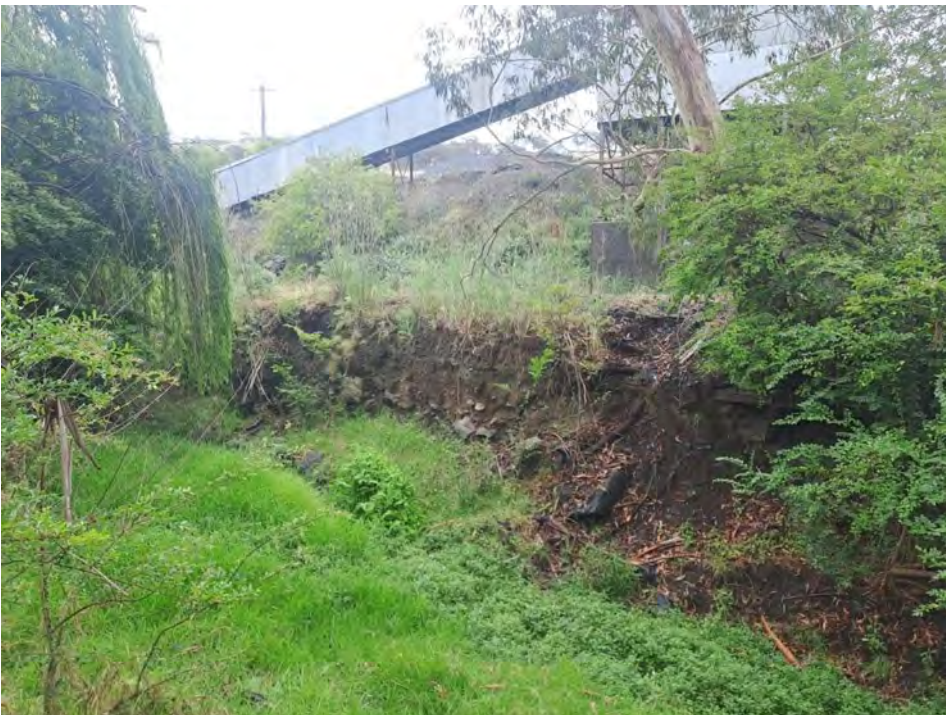
Photo 4.10 Creebank erosion along Doughboy Hollow Creek Study Area
