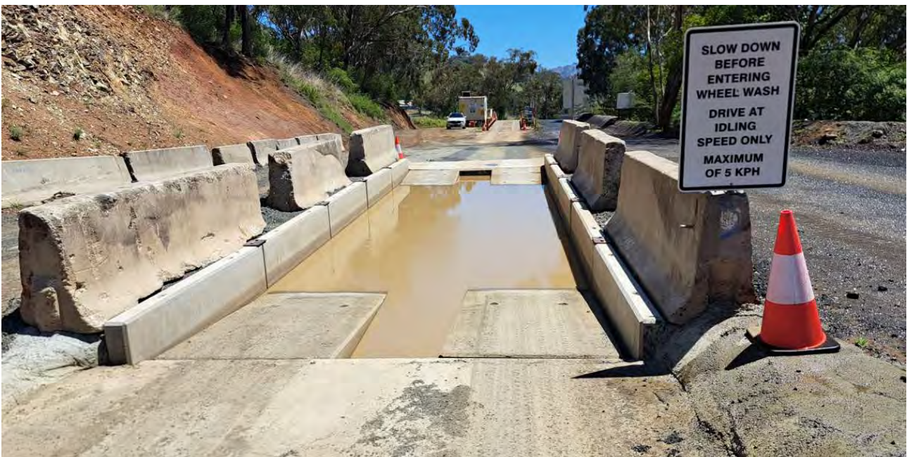
Photo 1: The new truck wheel-wash
